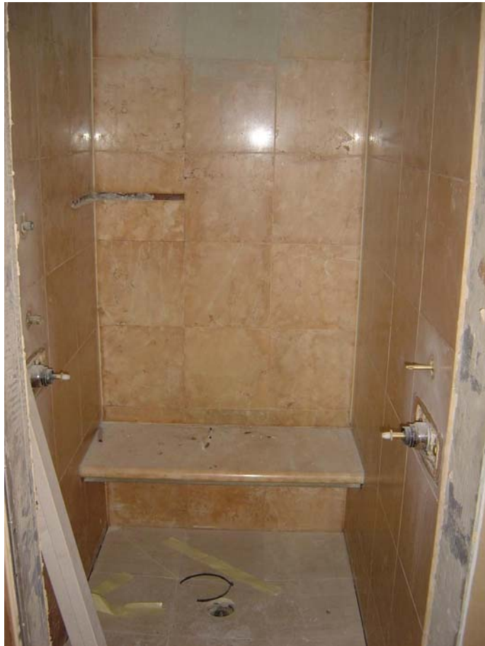
Old Shower Condition
